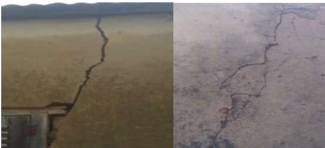
Figure 3. Cracks on the cement block wall.
